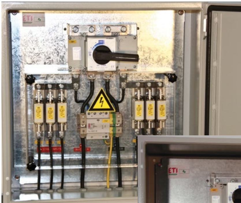
DC junction box (NH gPV fuses)
